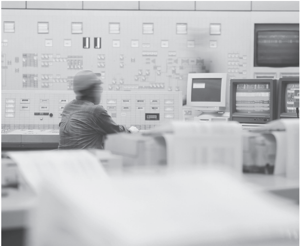
Figure 1.4 Typical industrial plant control room © Royalty-Free/Punchstock
